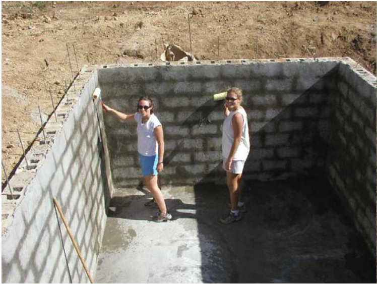
This new water cistern enables the orphanage to store water for irrigation use during the dry season.
