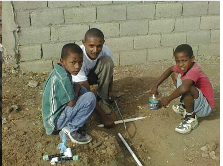
The boys helped to install a PVC irrigation system to move water from the cistern to the new garden and orchard.
